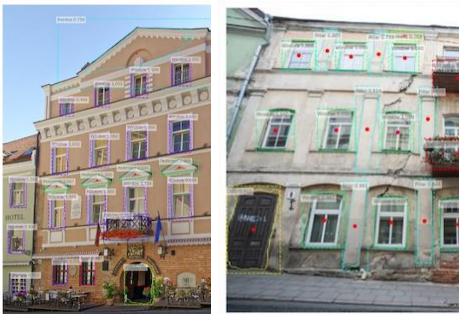
Fig. 7. The results of AI training: highlighted are different classes of objects identified by AI engine on photos taken at different angles towards the facade of a building
