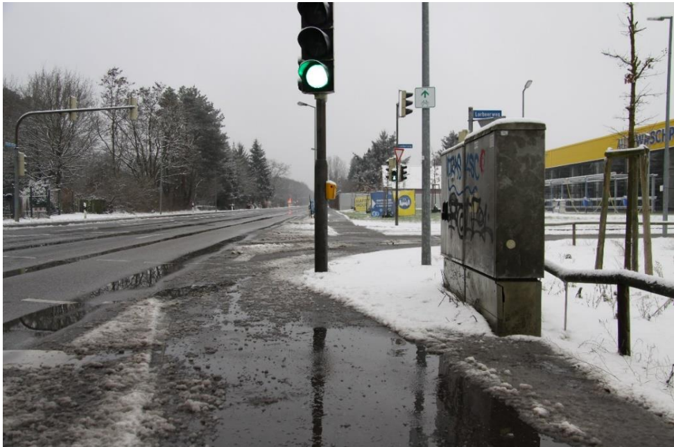
Fig. 2 – Difficult conditions on bicycle path for winter service because of infrastructure installations [picture source Cypra, 2021]
