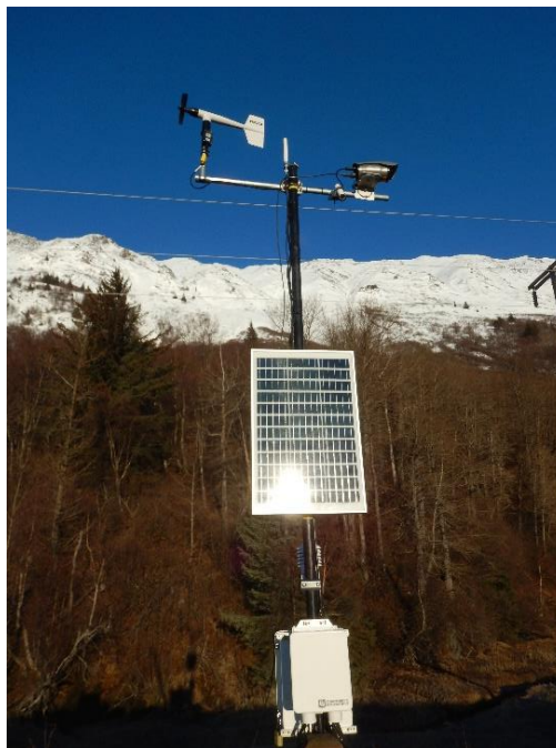
Fig. 1. mini-RWIS stations are self-sufficient, running exclusively on solar power and batteries to allow them to be placed anywhere you need them, regardless of existing infrastructure. They are easy to integrate, featuring embedded cell communication as well as NTCIP / Datex2 / Modbus compliance, making integration into an existing RWIS network simple.
