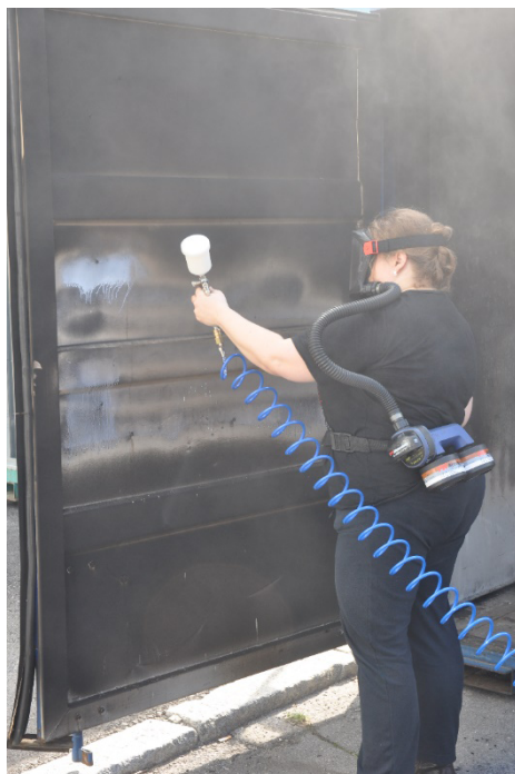
Figure 3. The application of liquid latex with a spray gun and a compressor system. Please note airway protection in the form of a respirator blower.
