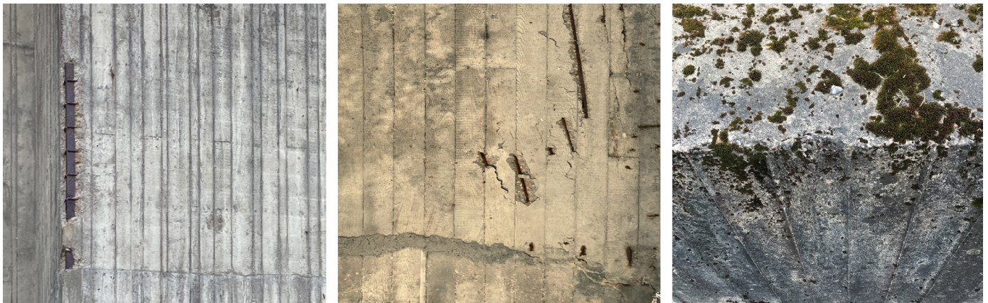
Fig. 5. Damaged raw concrete surfaces: on the left and in the middle – with opened reinforcement due to a thin decorative concrete layer; on the right – biological coating and sediments [photos by Aušra Černauskienė, 2019–2023].
